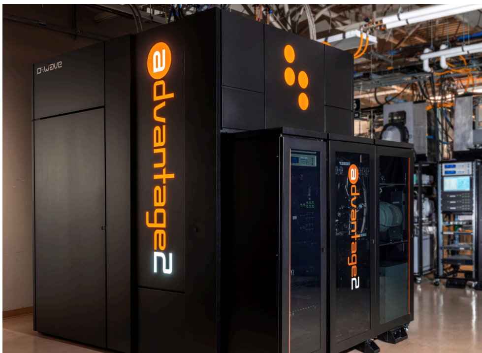
Figure 13: D-Wave Advantage2 quantum annealing system deployed in a facility. The system uses a closed-loop cryogenic dilution refrigerator, housed in a magnetic shielding enclosure, to maintain the QPU at its operating temperature below 20 mK.
