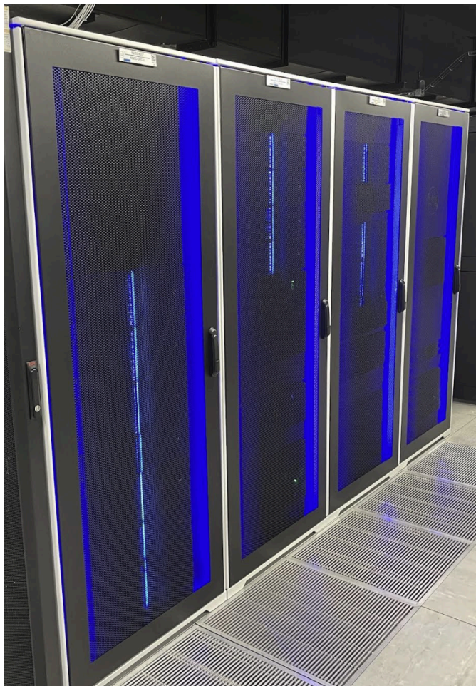
Figure 9: ORCA system deployed within a datacenter at the UK National Quantum Computing Center.
