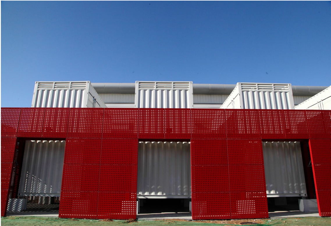
The indirect evaporative cooling module returns air through the ceiling from the upper part, exchanges heat with the outdoor cold air, and then sends air from the lower part back to the computer room. Therefore, it is very reasonable to put such module on the side of a large flat data center
