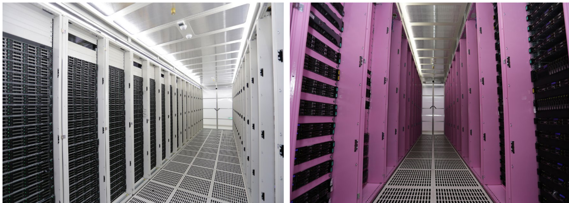
The cold aisles of different width in the ChinData Wangjing Data Center (the standard size of the floorboard is 600×600mm), which can be compared according to the stacking density of servers on the racks
