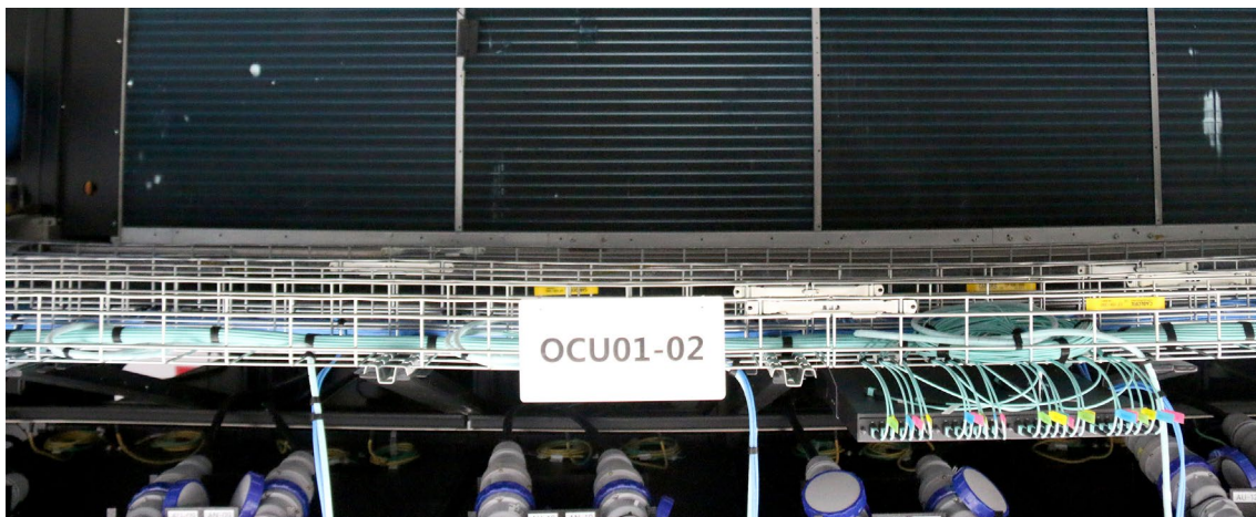
Air conditioner coil installed above the hot aisle (and rack)
