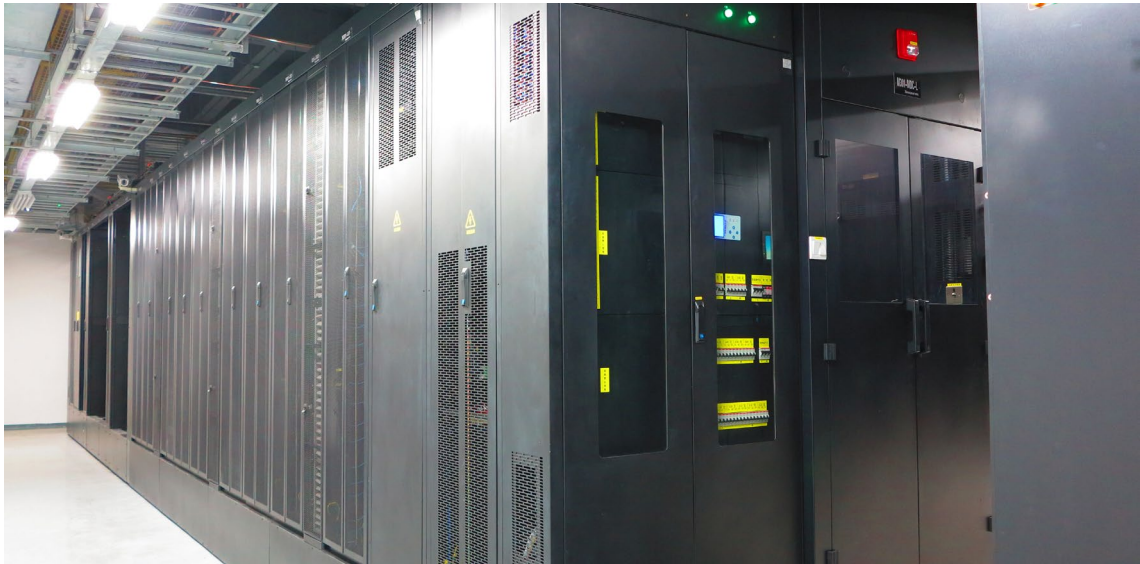
Wiring at upper part and water path at lower part for the micro-modules in the computer room of Tencent Tianjin Data Center (Source: Tencent Data Center)
