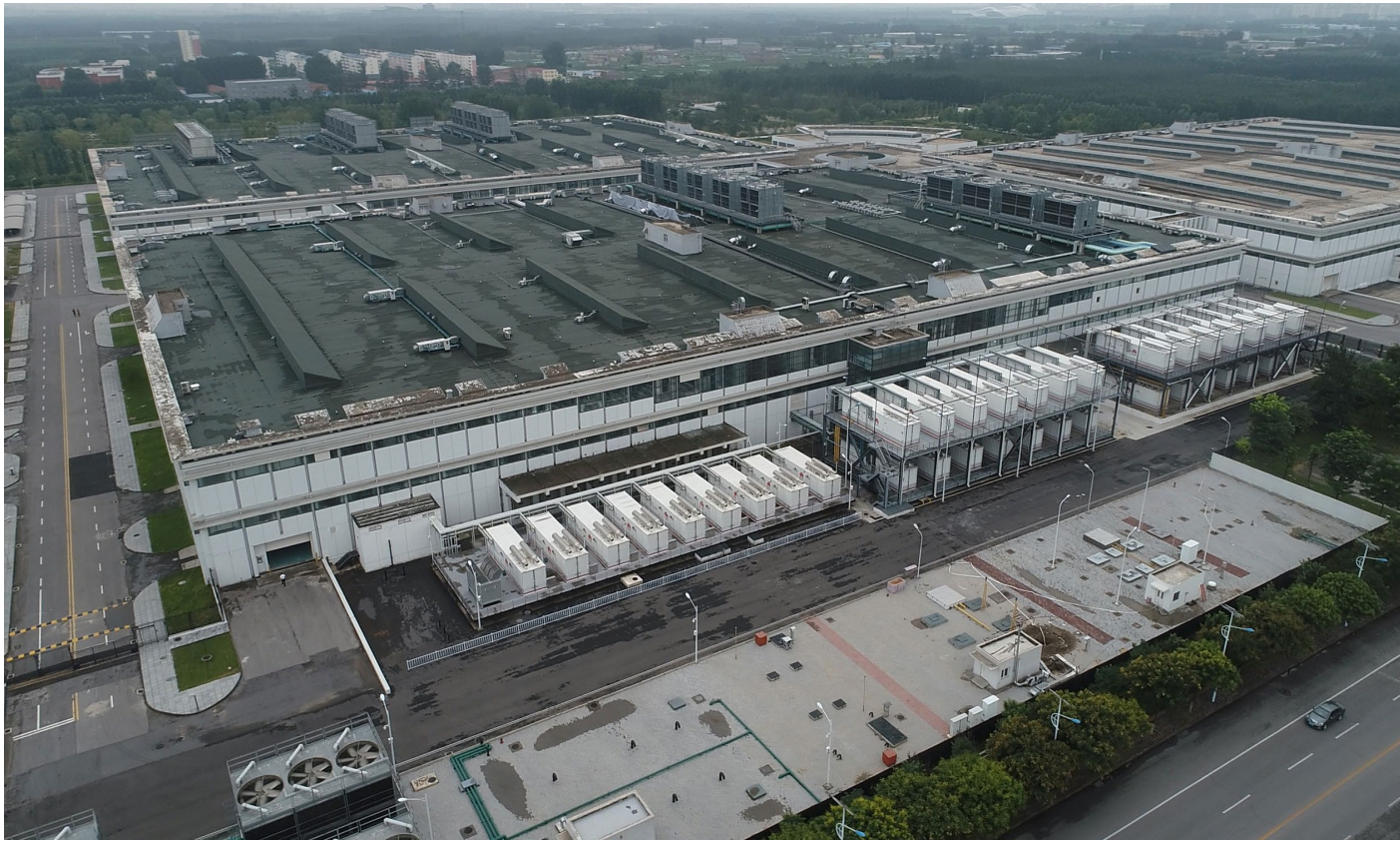
The diesel generators outside Huawei Cloud Langfang Data Center: 9 generators one set, and 7 for each of the other four sets, with a total of 37 generators. The gray ground across the road with diesel generators is the supporting oil depot
