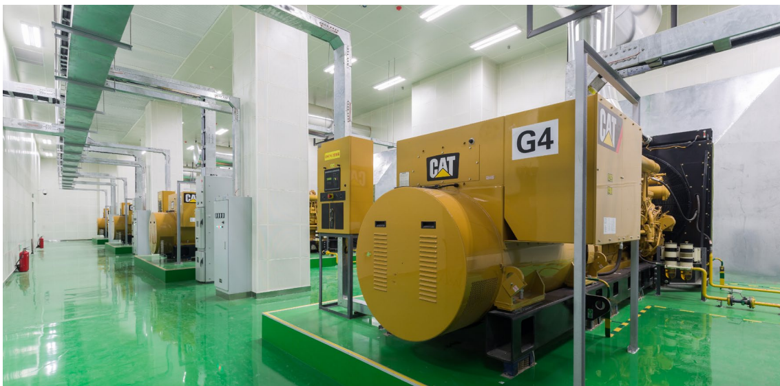
Diesel generator room of JD Cloud East China Data Center
