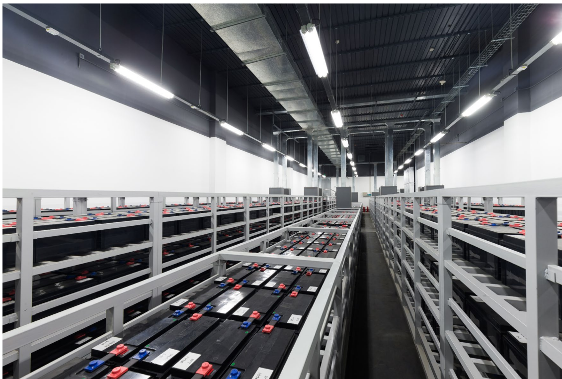
A battery room of JD Cloud East China Data Center (Source: JD Cloud)
