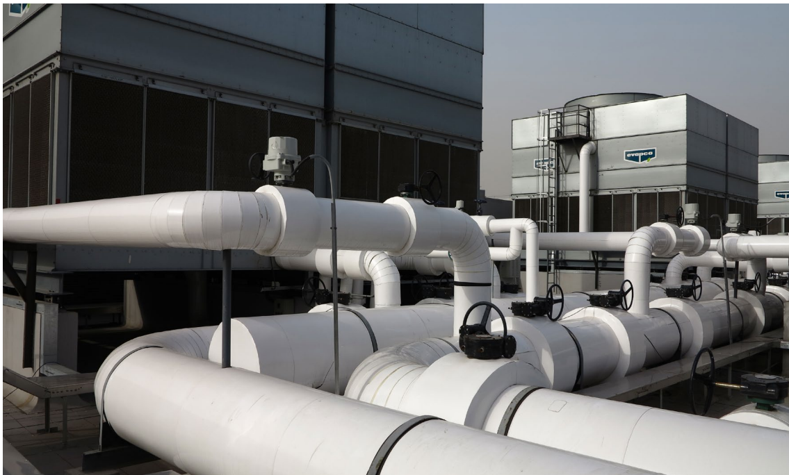
Cooling towers and water pipelines on the roof (Source: Tencent Data Center)
