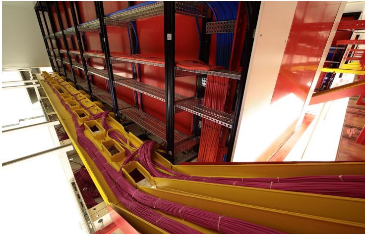
The ByteDance Huailai Data Center adopts the cable tray in the form of “gantry crane”, and lays different types of cables in layers (such as separation of two-source mains, power and control systems), and then enters the cable distribution frame installed in a way for short-depth rack at the IT rack’s upper part
