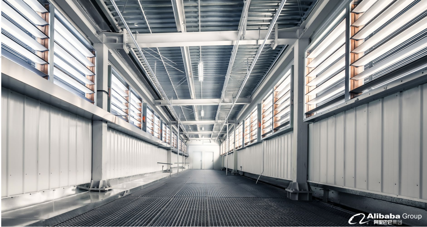
The inside of the roof attic area of Alibaba Cloud Zhangbei Data Center No.2 Campus - Phase I Project: please pay attention to the louvers on the left and right sides as well as the top light steel structure (Source: Alibaba Group)
