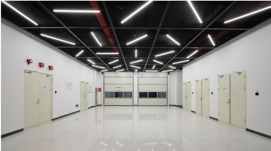
The spacious and bright server unloading and unpacking area is the goodwill of a data center for business
