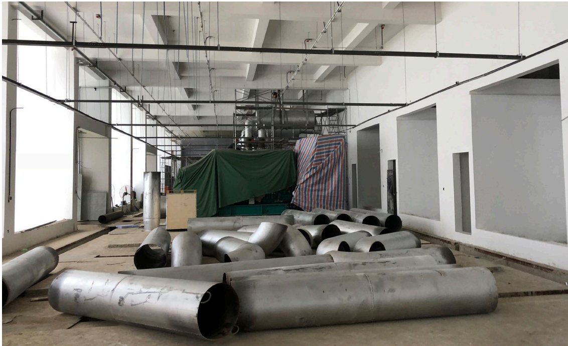
It is hard to guarantee the quality and progress of on-site construction
