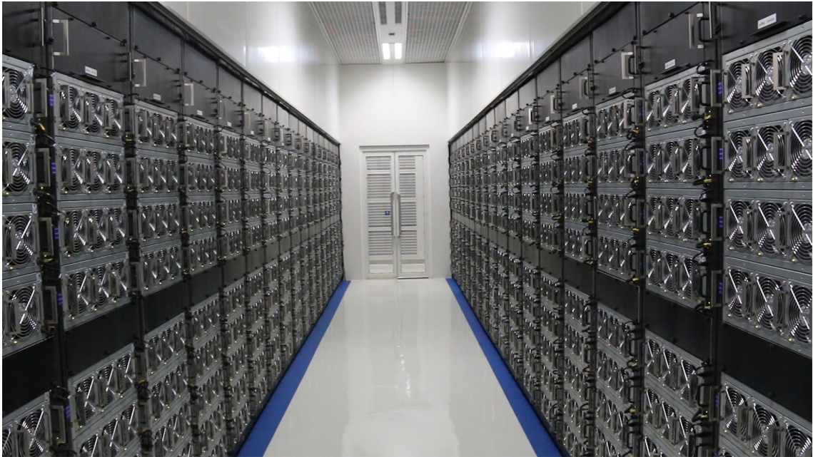
The hot aisle (containment) of computer room in Baidu Cloud Computing (Yangquan) Center, on both sides of which the back fan walls are built for the centralized cooling of North Pole 2.0 Rack servers
