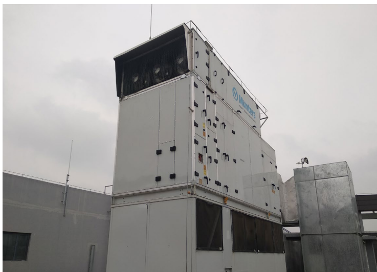
Indirect evaporative cooling module between the Module Buildings 7-8 of Baidu Cloud Computing (Yangquan) Center (Source: Baidu)
