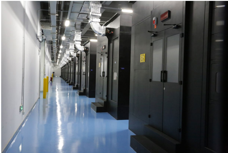
The most conspicuous feature of the first-generation warehouse-type micro-modules of Huawei is the design of single set cold and hot aisle containment
