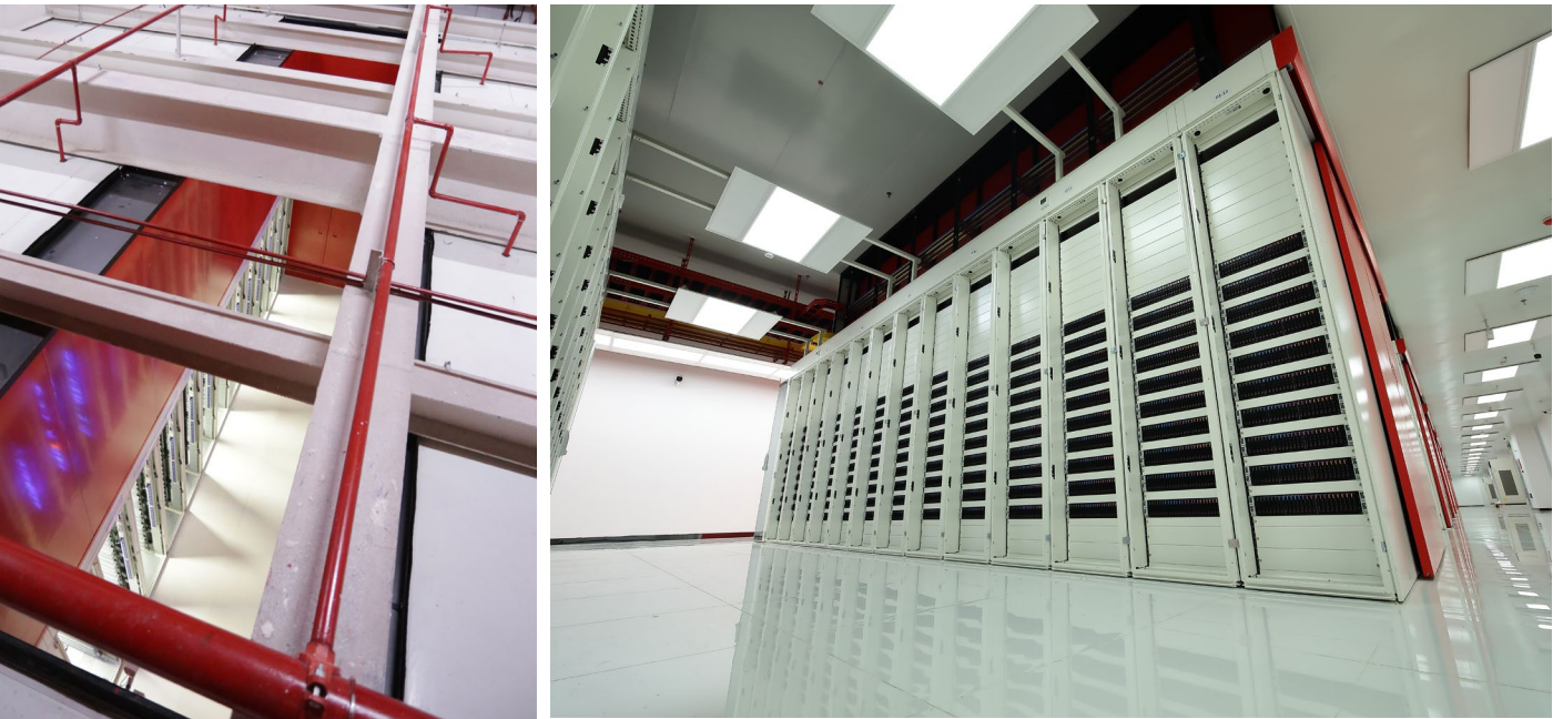
Standing on the ceiling of the ByteDance Huailai Data Center, you can see the hot aisle down.
