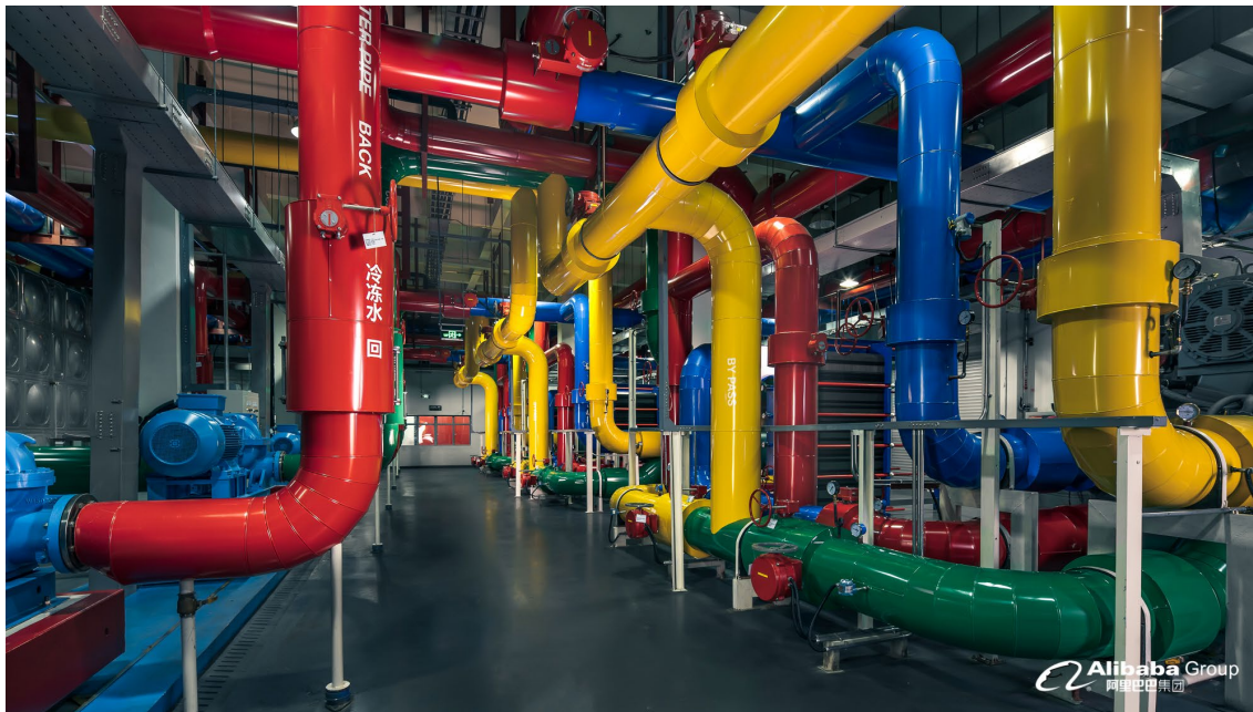
Interior of the cooling station in Alibaba Cloud Zhangbei Data Center (Phase I): the left side of the aisle is the water storage tank and the water chilling units of the chilled water system, and the right side is the plate heat exchangers and the cooling water pipes (leading to the cooling tower on the roof). Of course, the most attractive part is the various colors of the water pipes
