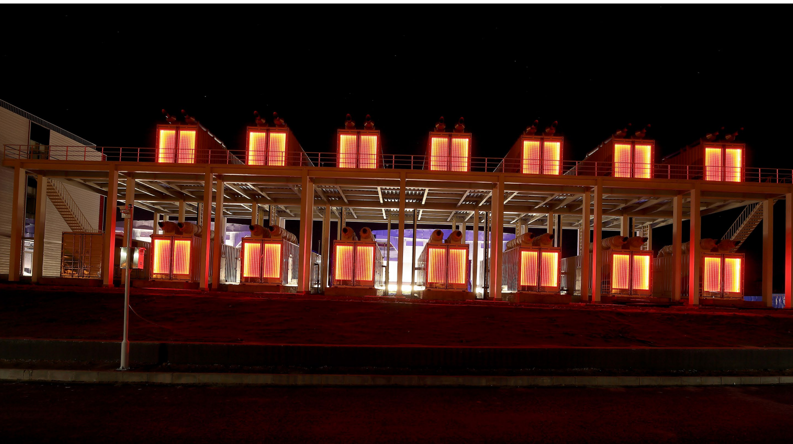
14 diesel generators of Phase I Project in ByteDance Huailai Data Center in use (regular drill)
