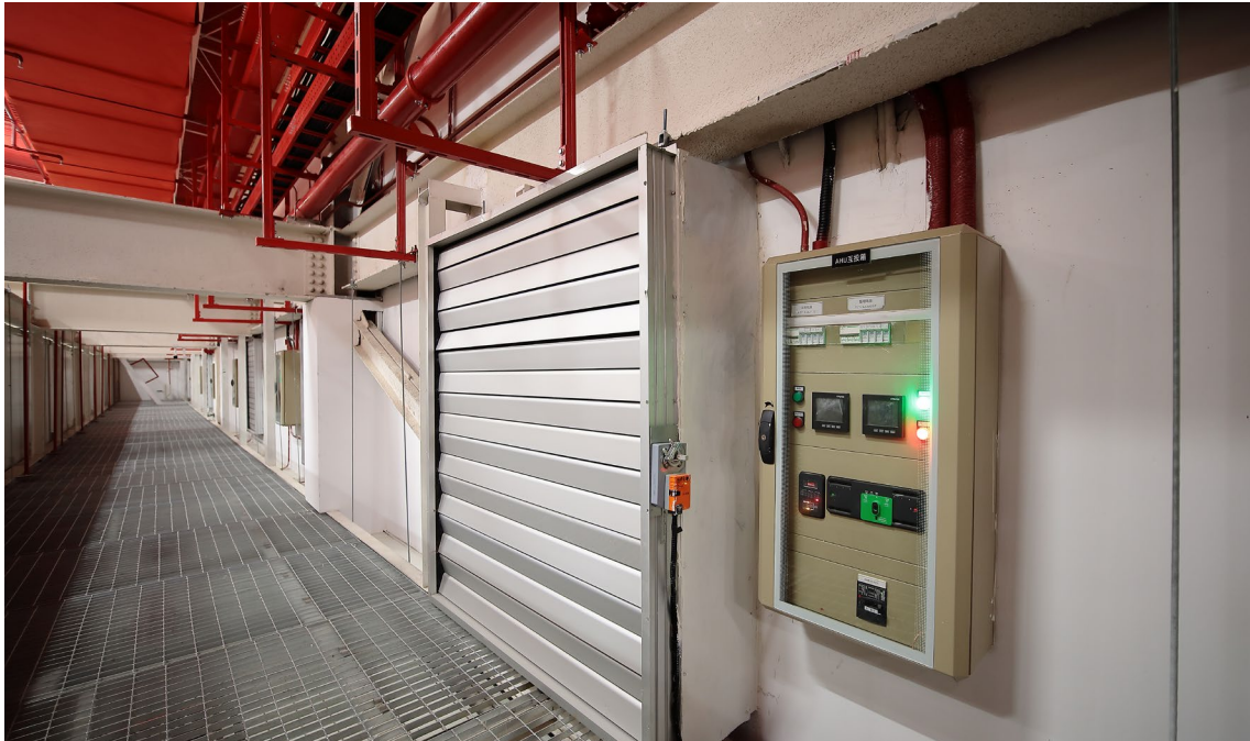
The return air inlet at one side of the ceiling above the computer room module in Phase I Project of ByteDance Huailai Data Center leads to indirect evaporative cooling module
