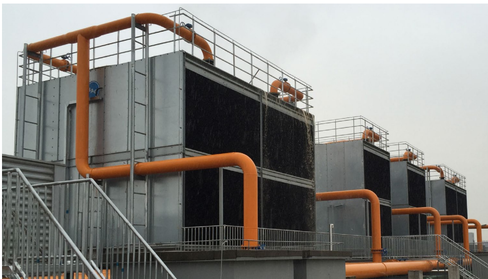
Cooling tower in operation
